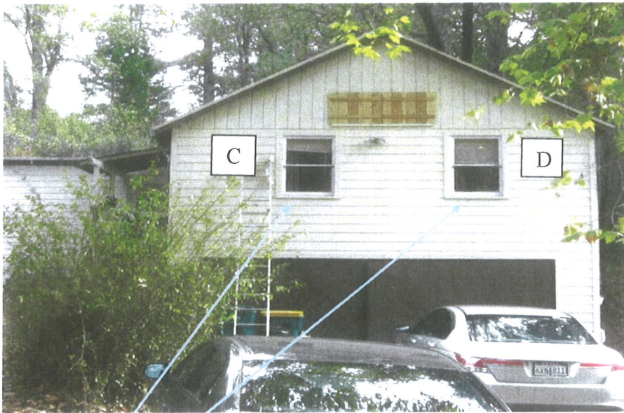
Windows C and D...single hung, single pane, wood sash, size 30" x 48", both windows are in poor non-operable condition.
